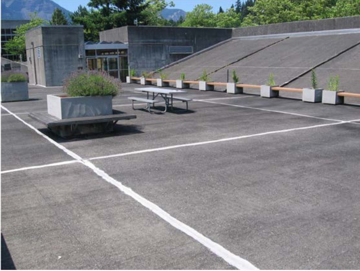
Photo 2. Close up of the roof area to be repaired and the caulking to be removed.
